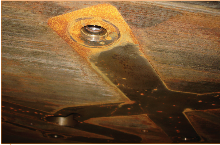
Inspect for leakage, kinks, cuts and restrictions that can cause a water leak, as seen inside this hot half assembly.
