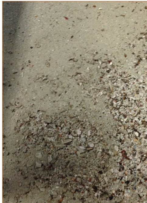
A combination of scale, rust and organic materials was collected from an open-loop cooling tower.
